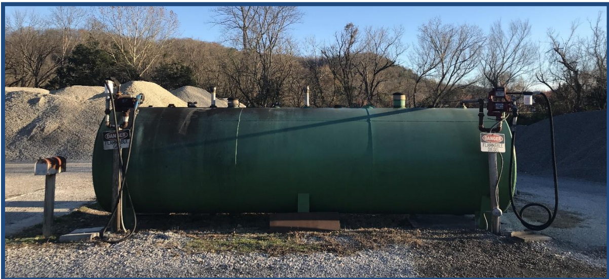
Fuel tank located at the department, including the diesel fuel nozzle (left) and gasoline fuel nozzle (right)
