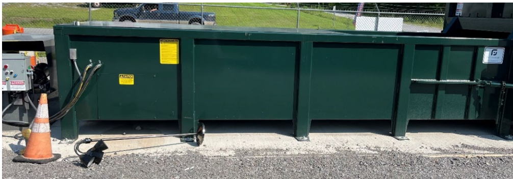
Concrete pad poured by the county commissioner in July 2024 at the county convenience center
